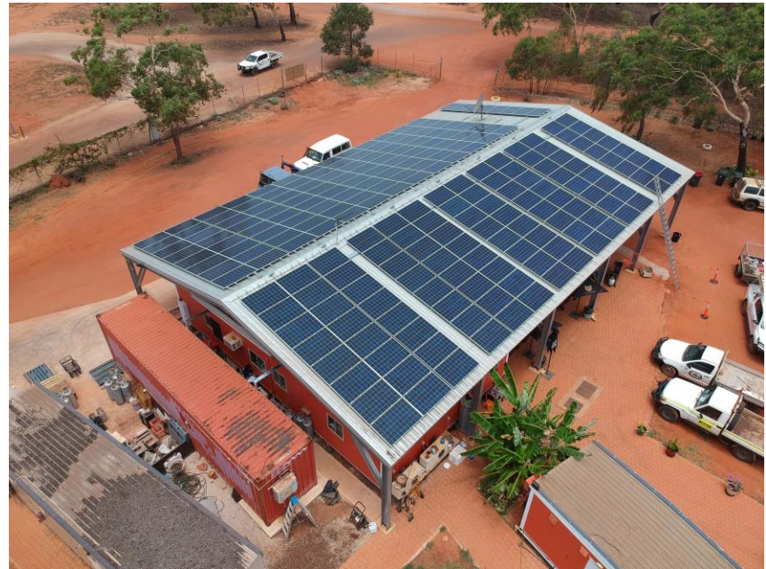
Source: West Australian Alternative Energy - Djarindjin Corporation partnering with Horizon Power as part of the Solar Incentives Scheme. Under the Scheme
